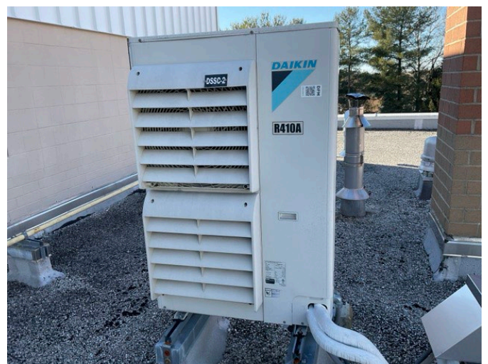
30 - SPLIT SYSTEM DUCTLESS
