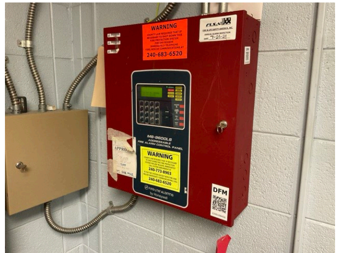
34 - FIRE ALARM PANEL
