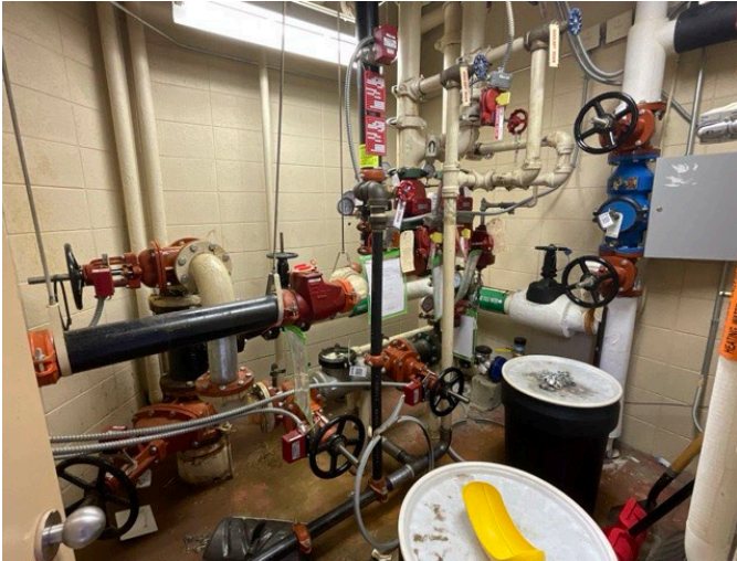
31 - FIRE SUPPRESSION SYSTEM
